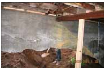
City building inspector investigates a residential eroding basement wall
