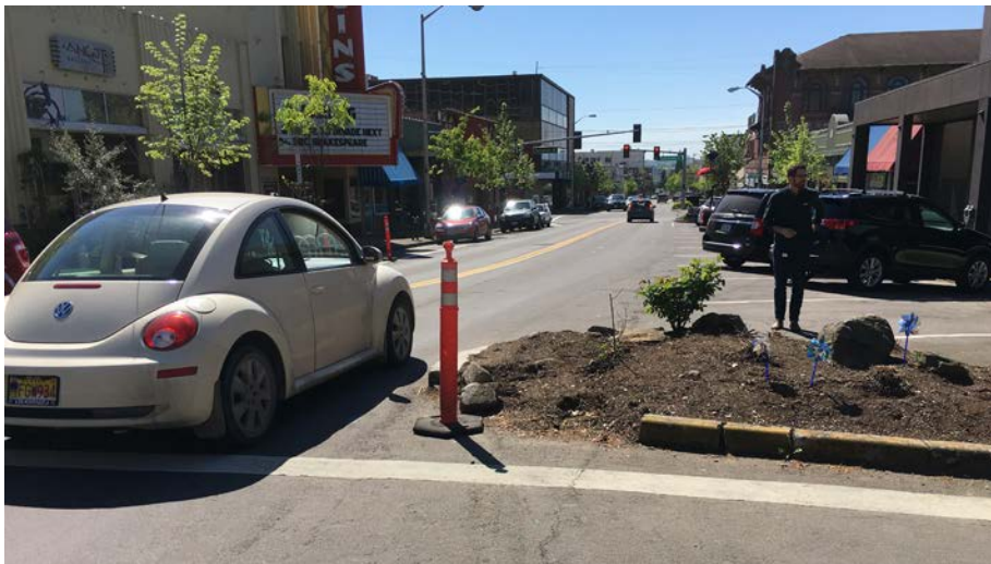
The inconsistent and deteriorating streetscape of Main St. in downtown detracts from the street's ability to support a thriving retail district
