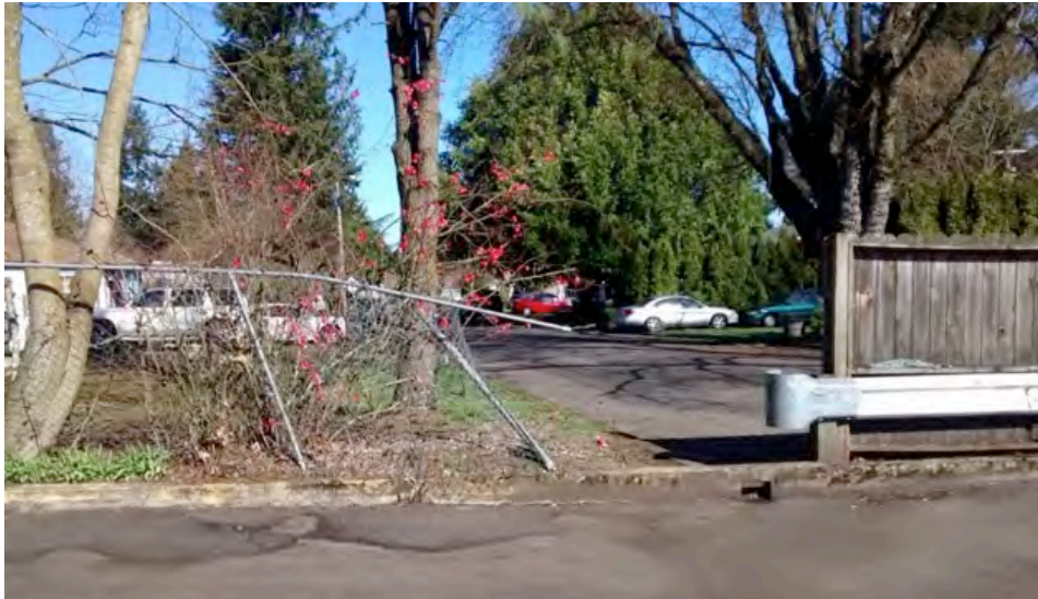
Pedestrians may create their own connections to bypass a circuitous street network. These connections can be formalized to improve safety and make them accessible to people of all ages and abilities
