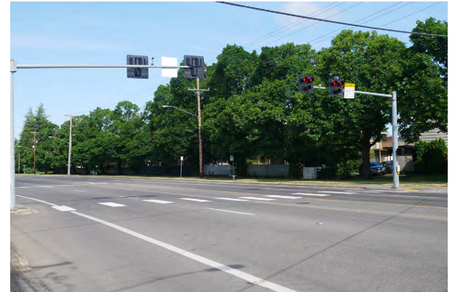
Pedestrian Activated Signal
