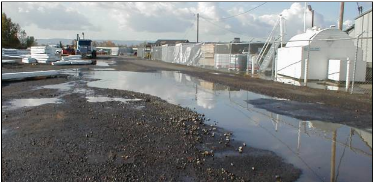
Figure 9 - Standing water along 2 nd Street after rainstorm
