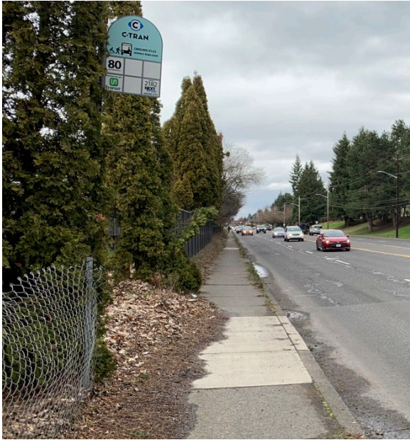
Photograph 2-16. Bus Stop Lacking a Shelter and with Debris on the Sidewalk
