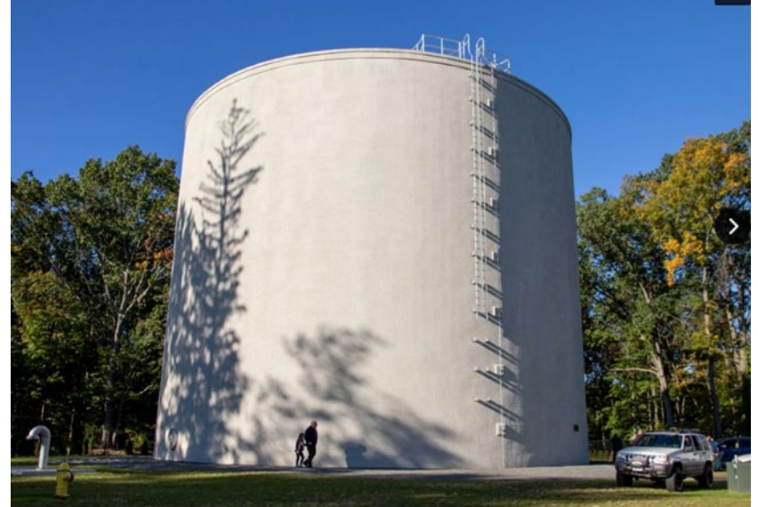
2 M gallon tank
