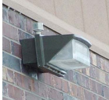
Bad: Unshielded wall box Dept of Health (Town Center East)
