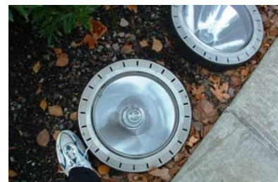
Metal halide flagpole lights DOT Bldg (Linderson Way)
