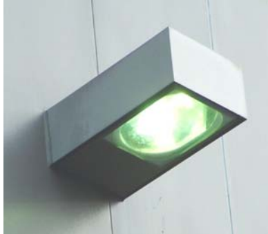
Good: Fully shielded wall box WA Dept of Printing (New Market St.)
