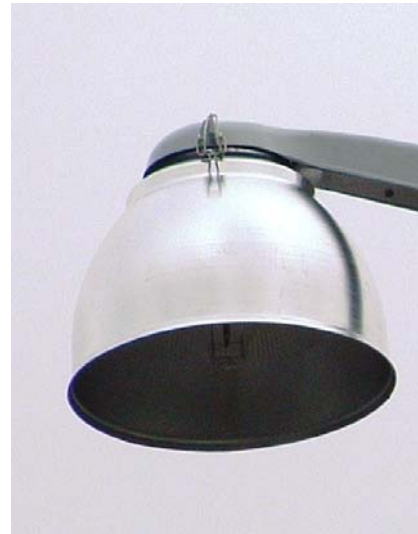
Shielded version at former State Parks & Rec Bldg
