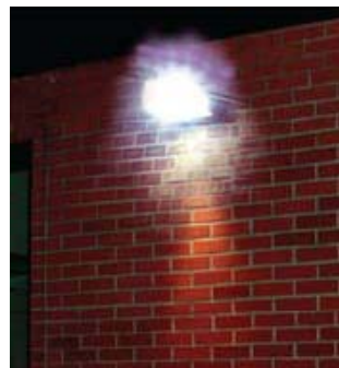
Unshielded wall box
