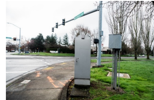
Figure 36 Example of a Traffic Signal and Traffic Signal Controller
